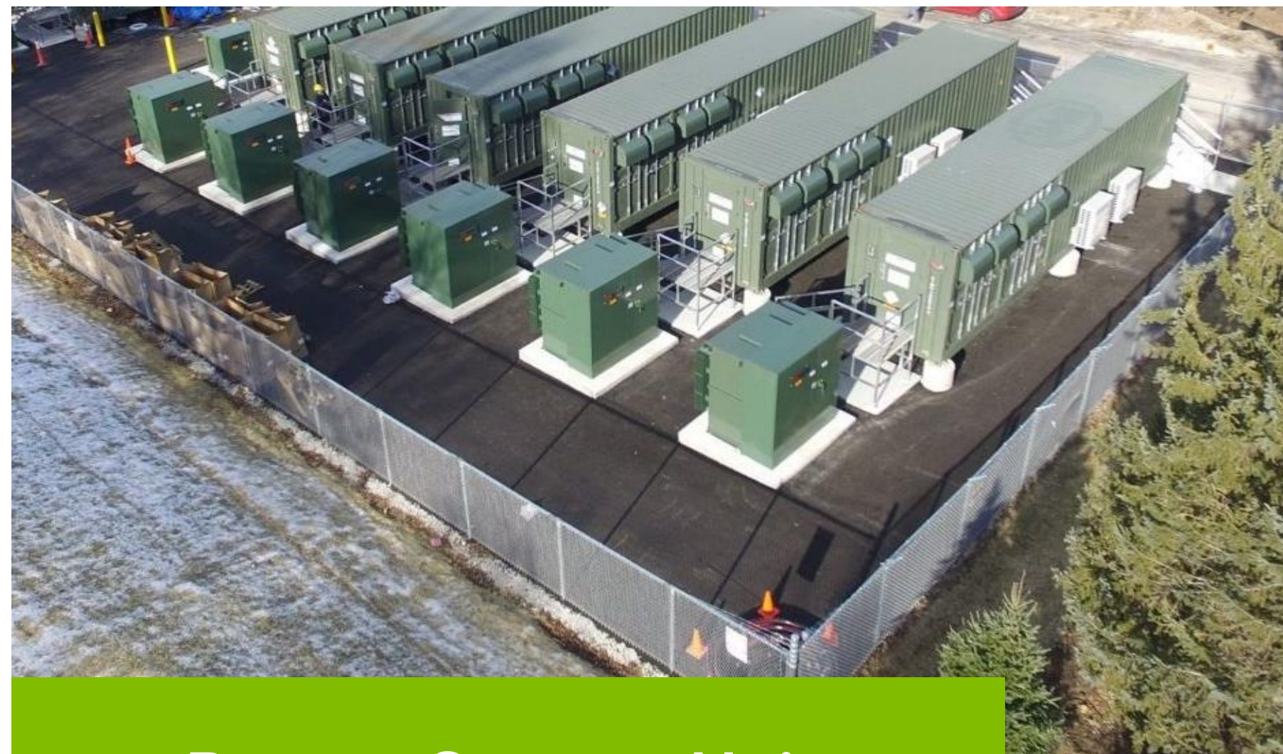
Battery Storage Units
