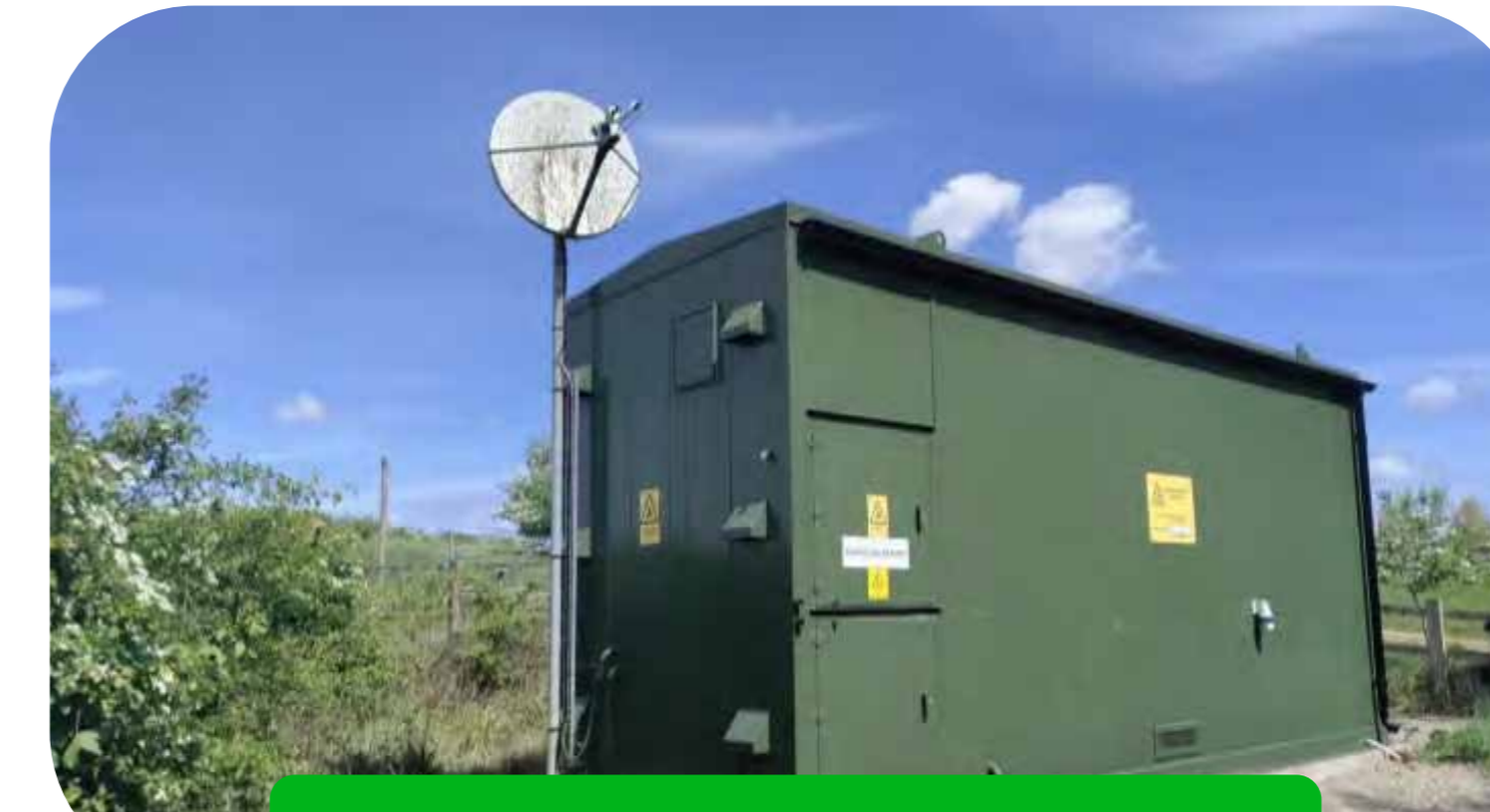
Switch Gear Cabins
